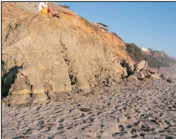
Character Sample Rock E Rock boulders and deeply eroded rills are common
