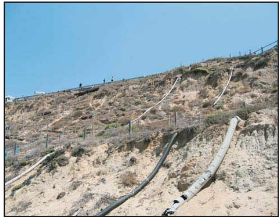
Visual Character Unit 1b Project Site Slope Exposed Pipes
